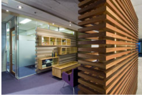
Recycled timber return air screen at entrance to Zero Waste SA office.
